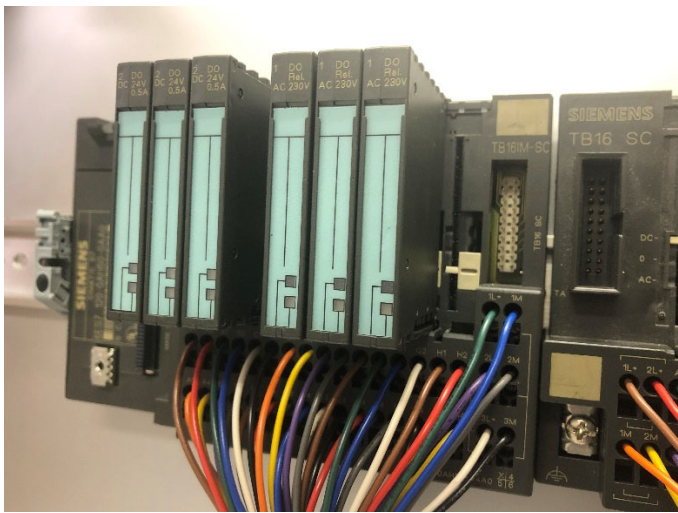
Existing ET 200L-SC IM-SC system
